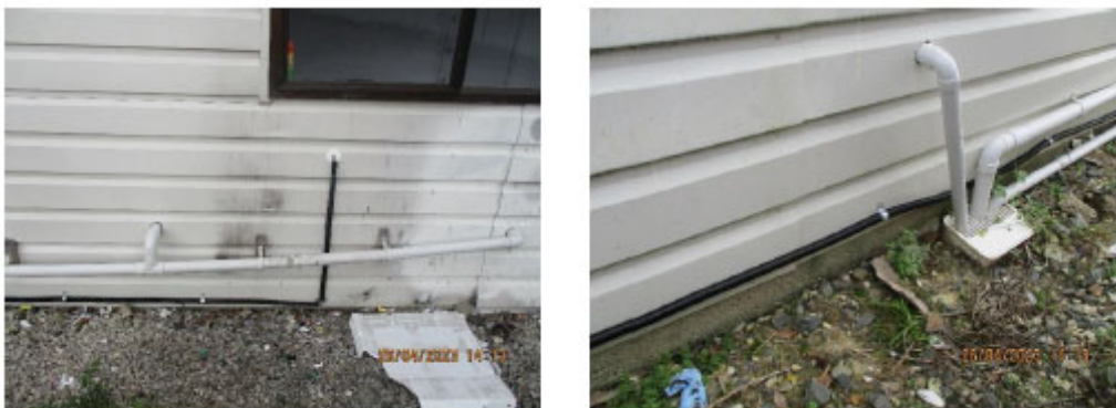
Figure 2. Photographs from the second inspection, captioned “Gas pipe raised above ground, covered with conduit and clipped”.
