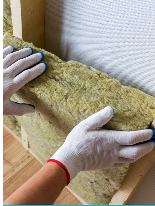
Retrofitting or installing thermal insulation in external walls of a standalone dwelling under certain conditions
