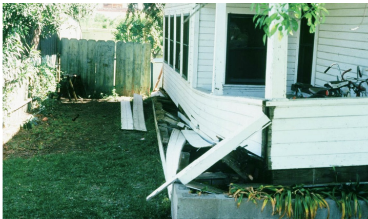
Figure 11: House fallen off its foundations
