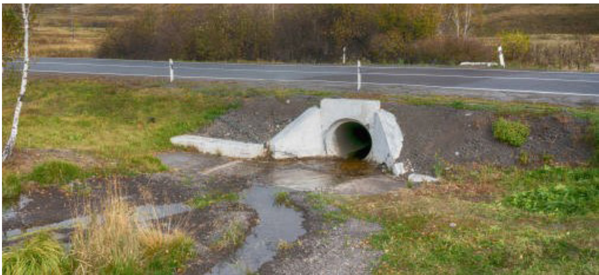
Figure 3: Hillcrest Road at Tau Creek culvert. (Source: Heathcote Regional Council)
