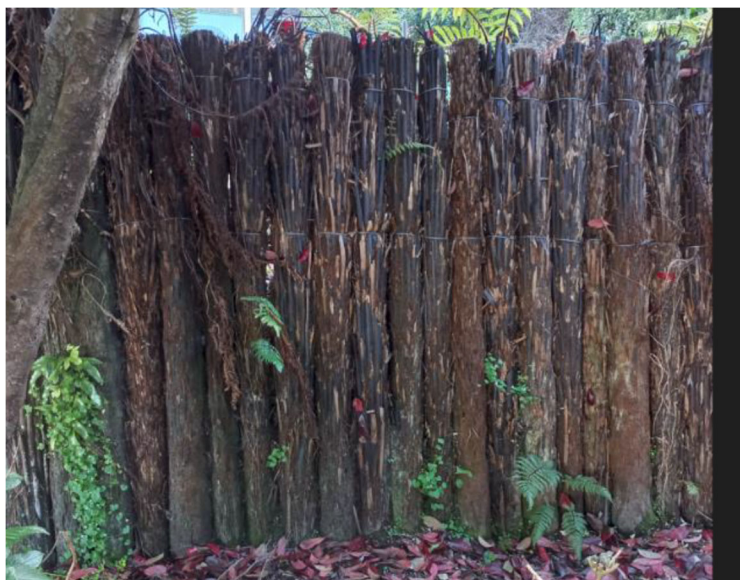
Figure 3: Photograph of the new ponga wall (5.6m long and 2m high), from the neighbours' side, provided by the authority
