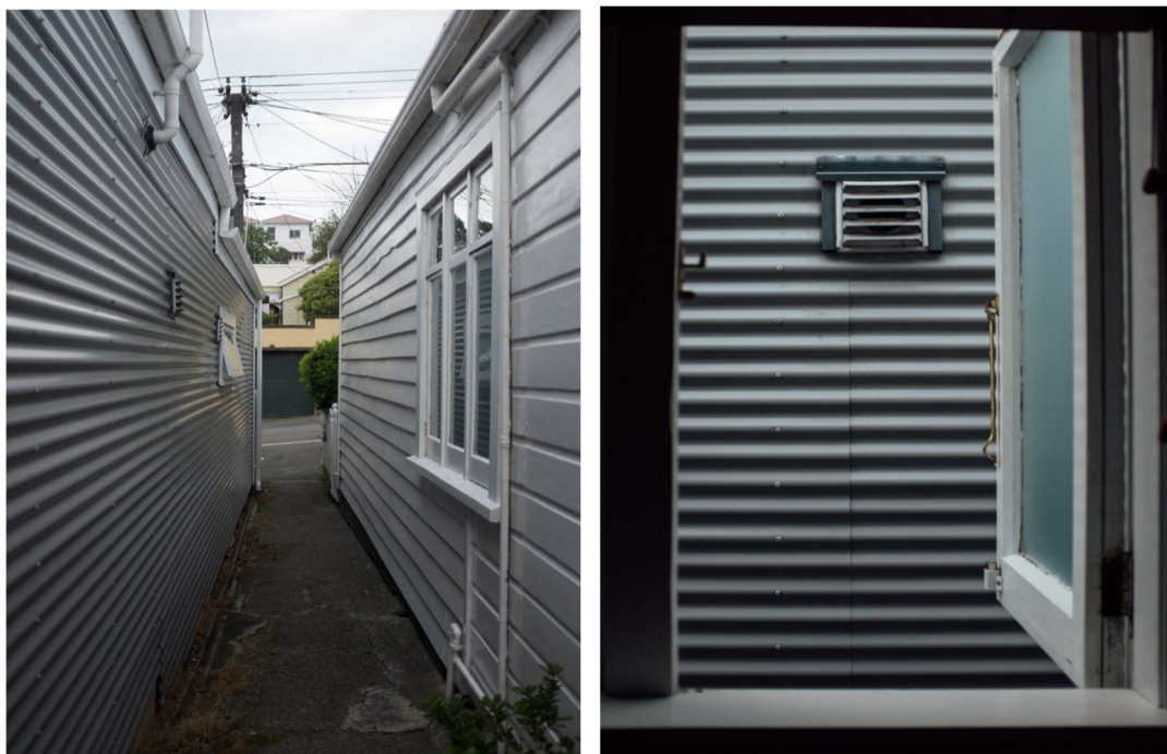
Figure 1. Location of the exhausts from the ventilation system in relation to the neighbour's entrance pathway and living room window.
