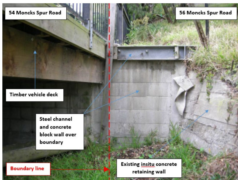
Figure 5: View looking south at encroachments over boundary
