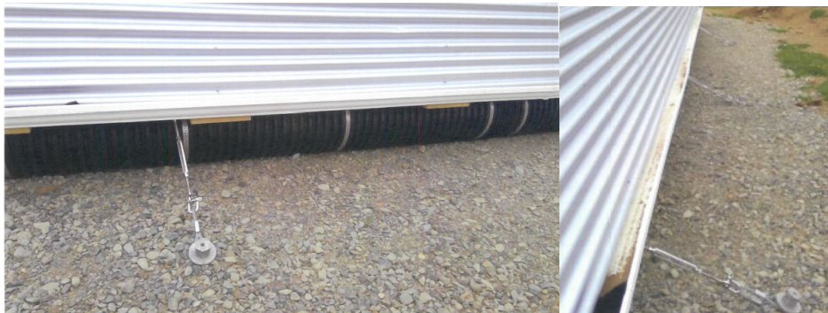
Figure 4: Photograph showing a pontoon and earth anchor (left) and earth anchors located on the side of the dwelling (right). Note the angle of rigging screws and anchors.
