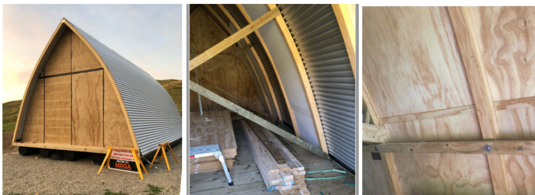
Figure 2: Photos showing construction of the roof, including the corrugated iron sheeting (left), curved frames and polystyrene insulation (middle) and internal plywood lining (right).
