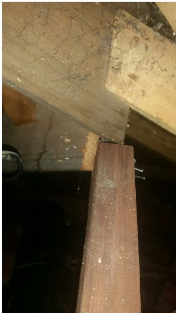
Photo 3. Top of strut with nails present and no observable splitting in the timber.
