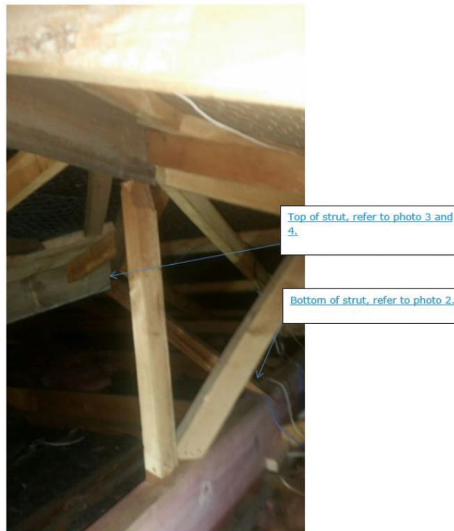
Photo 1, showing the strut which has been noted as being poorly installed.
