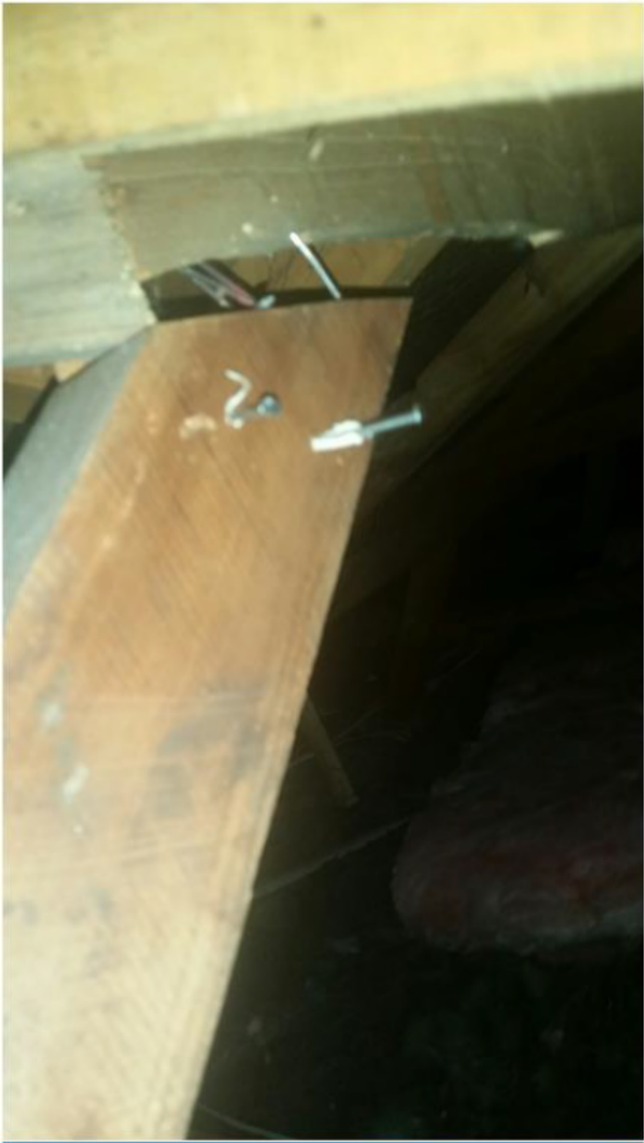
Photo 4, Top of strut with no observable splitting of the timber as installed.
