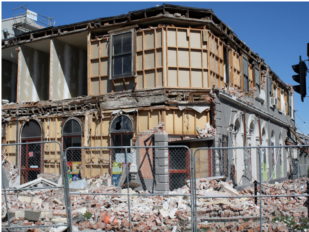
Figure 2: Collapse of the facade of a two-storey building in Christchurch, February 2011.
