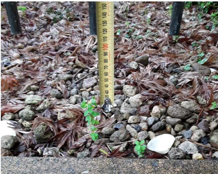
Figure 5: Gaps between fence and pebbled garden
