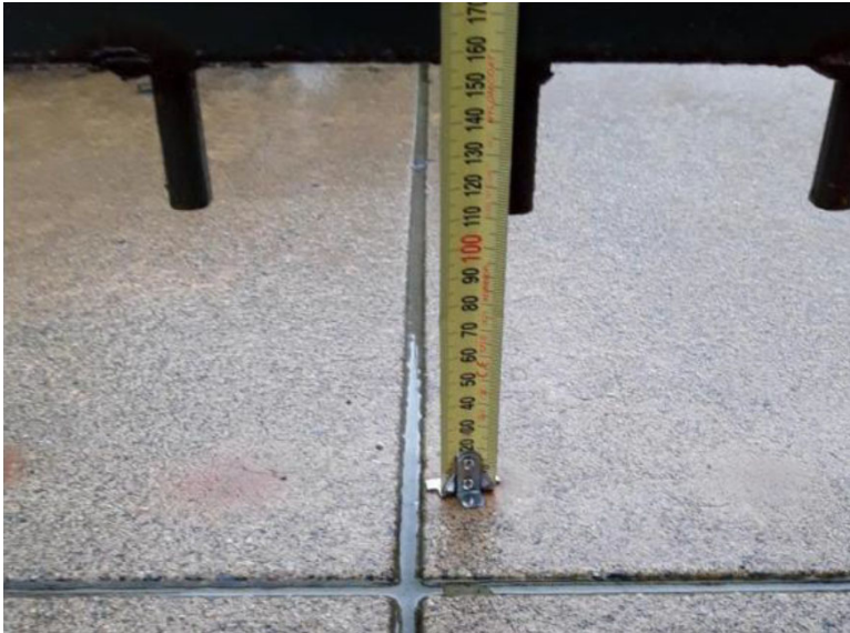
Figure 4: Gaps between fence and paving
