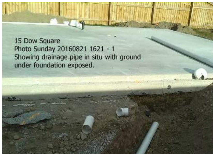
Figure 1: Detail of ground and foundation on 21 August 2016 (image supplied by the applicant)
