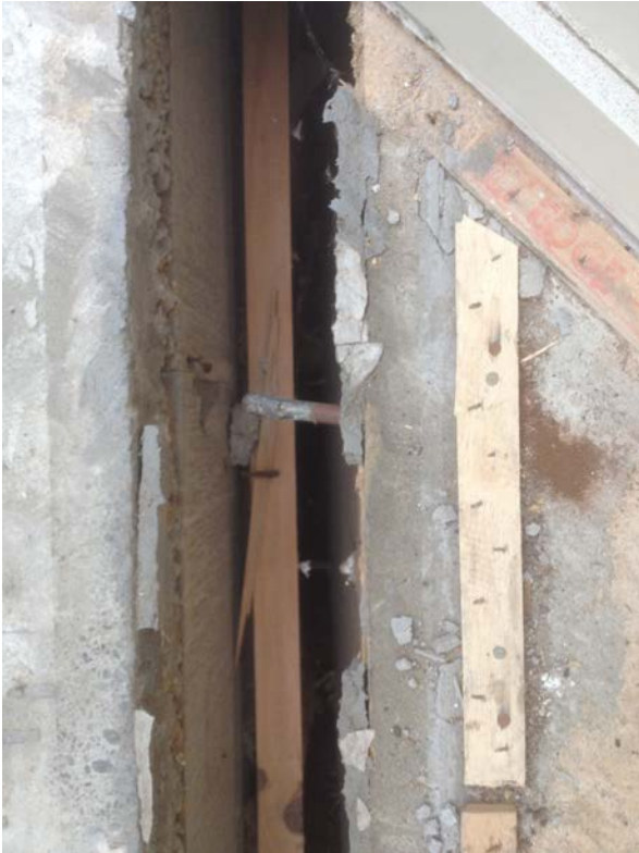
Figure 5: Rupture at interface between single and two storey parts of house
