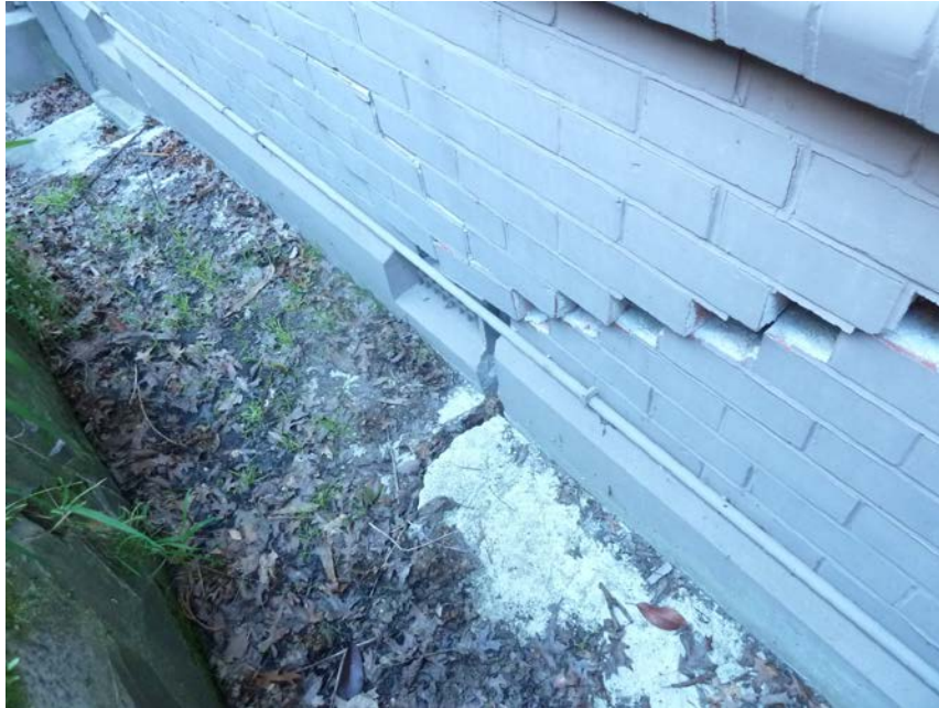
Figure 7: Rupture of concrete foundation beam and brittle cladding
