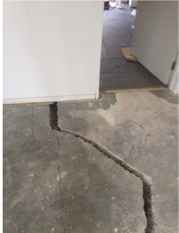
Figure 6: Rupture of concrete floor slab
