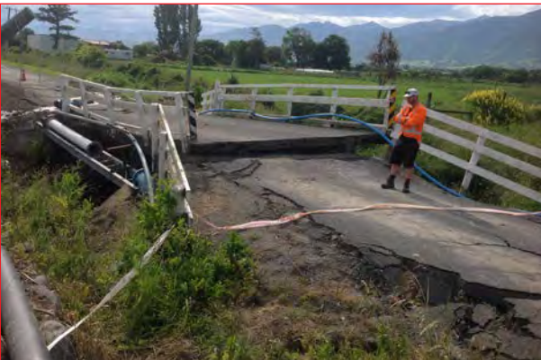
Bridge damaged by lateral spreading
