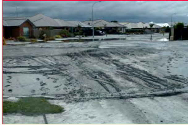
Liquefaction ejecta in turning circle of Seabreeze Close
