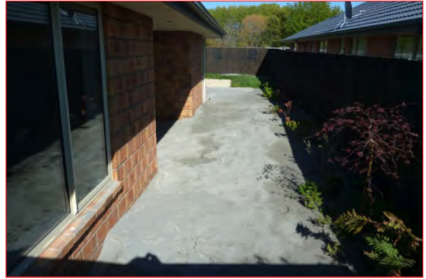
Large amounts of liquefaction ejecta
