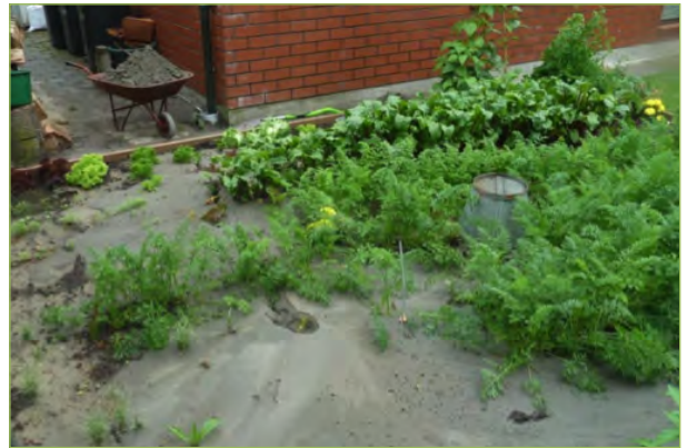
Liquefaction ejecta in planter
