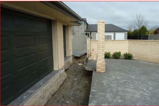
1 m wide crack from lateral spreading
