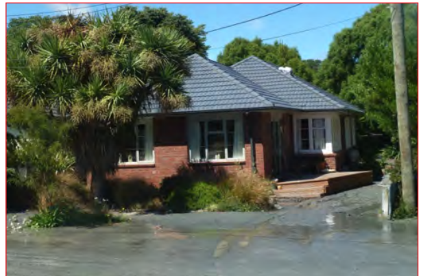
Foundation damage, tilting dwelling
