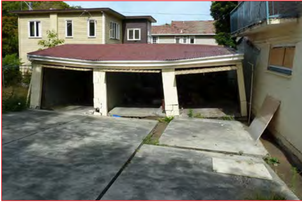
Drive and garages deformed by lateral spreading
