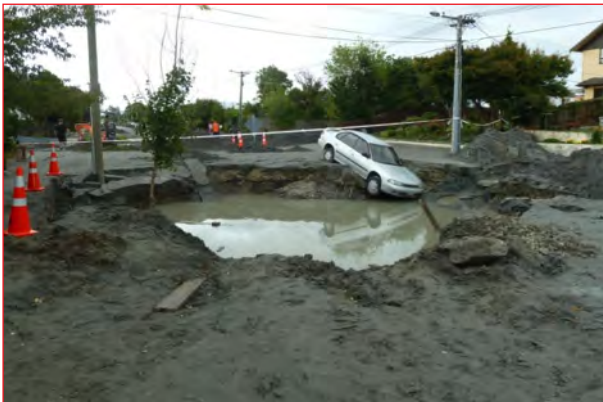
Close up photo of road damage seen in aerial photo of Woolston
