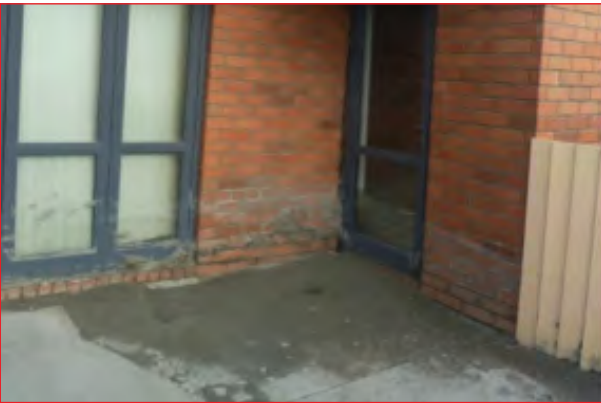
Outside of dwelling showing level liquefaction ejecta reached on brickwork and windows
