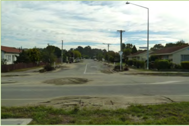
Liquefaction ejecta at a New Brighton Road junction
