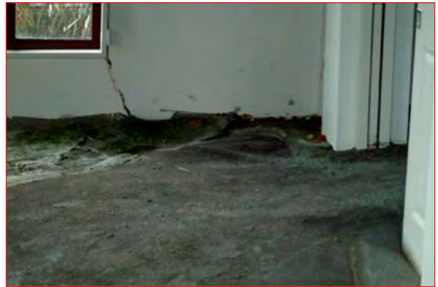
Large amounts of liquefaction ejecta inside dwelling
