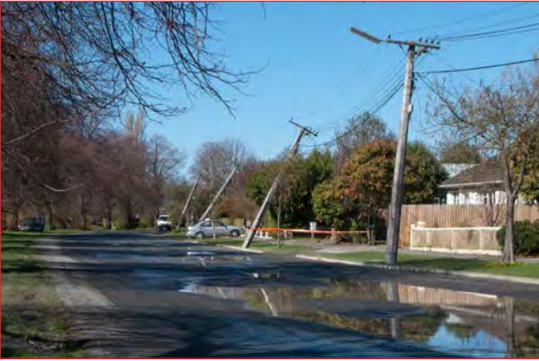
Lateral spreading damage to power lines
