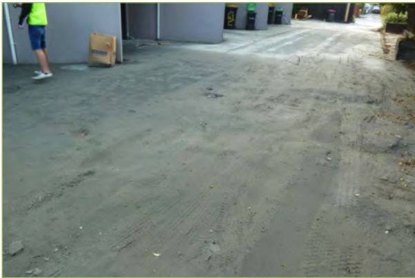
Liquefaction ejecta covering driveway
