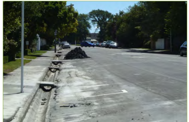
Liquefaction ejecta pile on road
