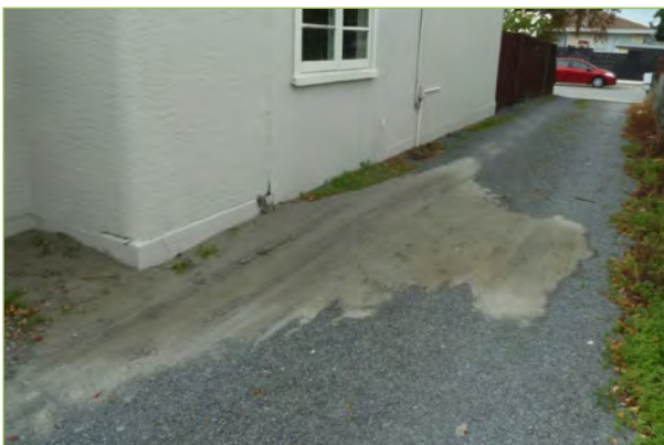
Isolated area of liquefaction ejecta
