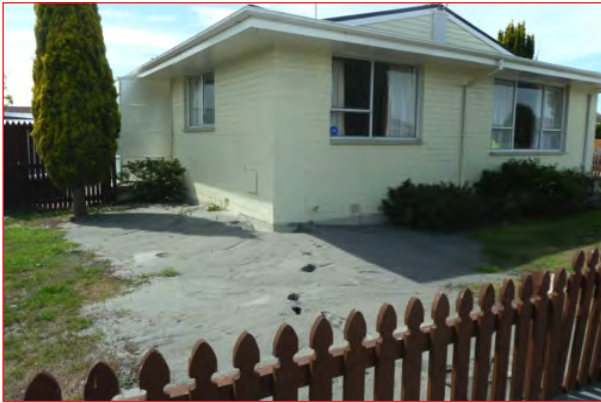
Large patch of liquefaction ejecta
