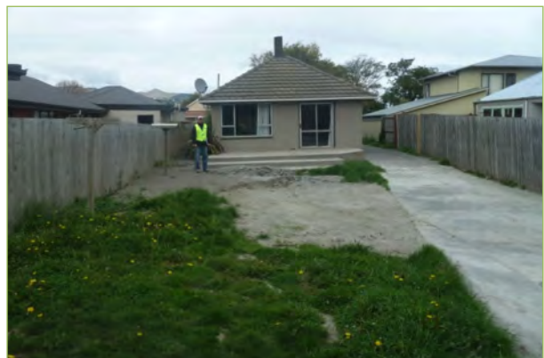
Liquefaction ejecta, dwelling tilting
