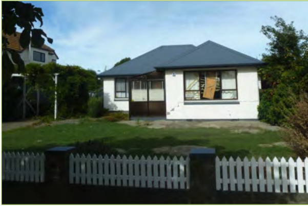
Liquefaction ejecta in many areas on lawn
