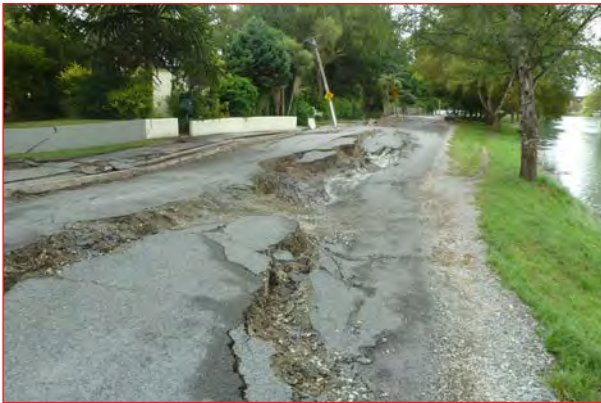
Lateral spreading damage to road and powerlines
