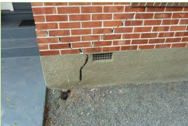
Foundation and brickwork damage
