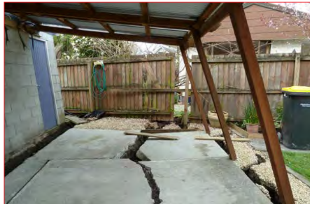
Carport pulled apart by lateral spreading
