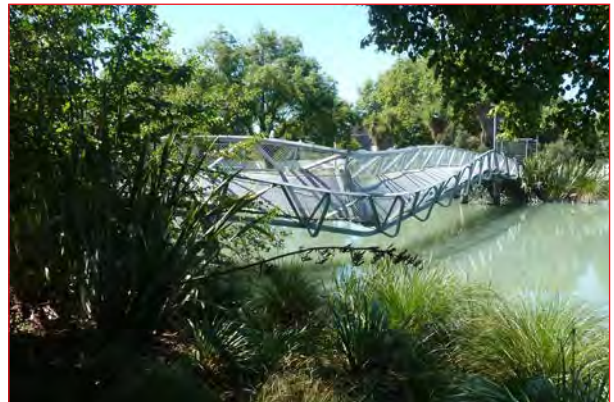
Buckling of bridge caused by lateral spreading
