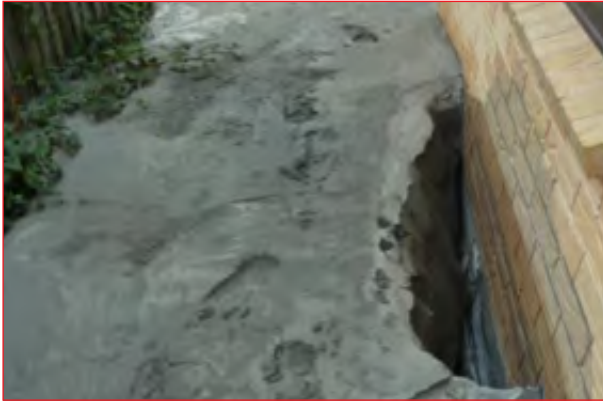
Large amounts of liquefaction ejecta
