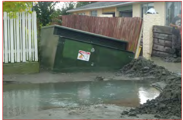
Power substation punched into ground
