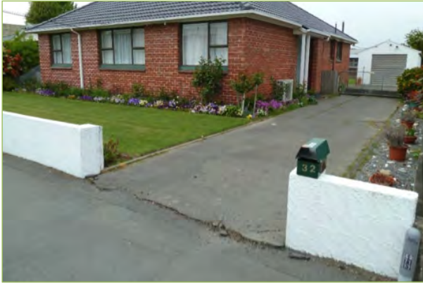
Damage to asphalt
